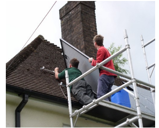
PV panels being installed on the roof of Jon Cooke's bungalow. 14 panels were installed by Greenerth Energy in June 2007
